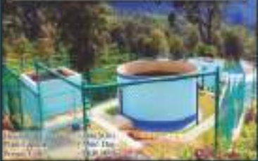
Bogawana Water Supply Scheme
